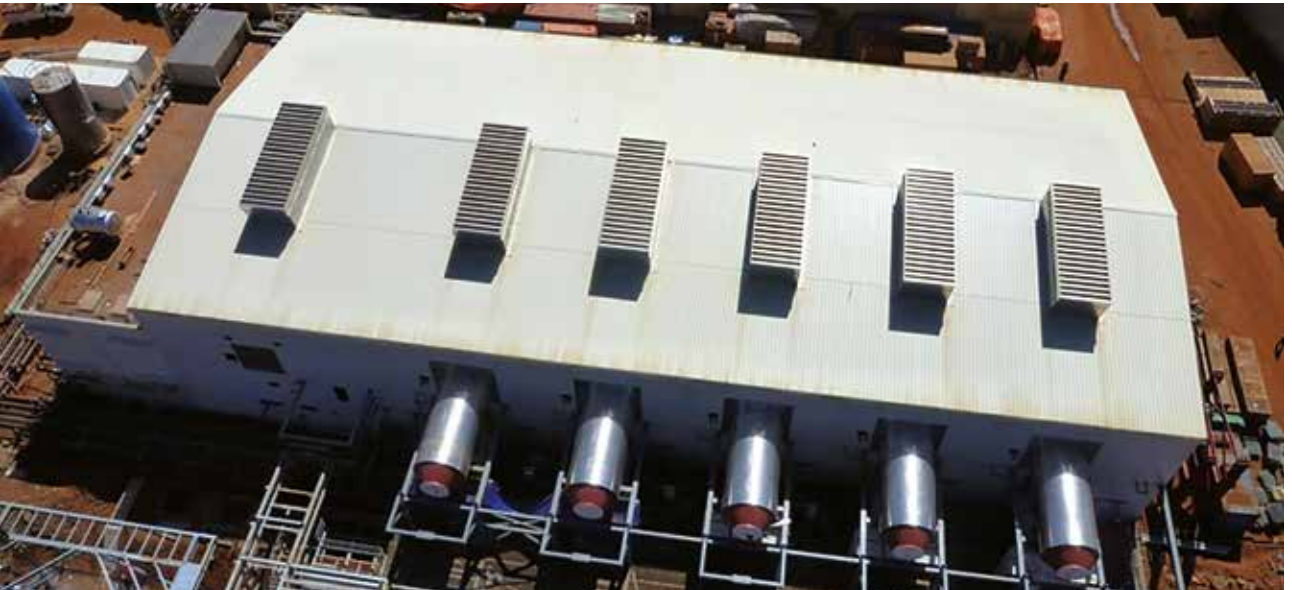
Thika Power Plant - Kenya / Taşyünü Cephe Paneli
