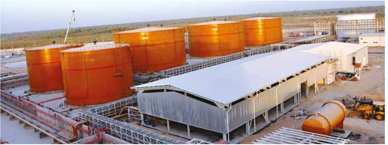
Nainawa Power Plant - Irak
