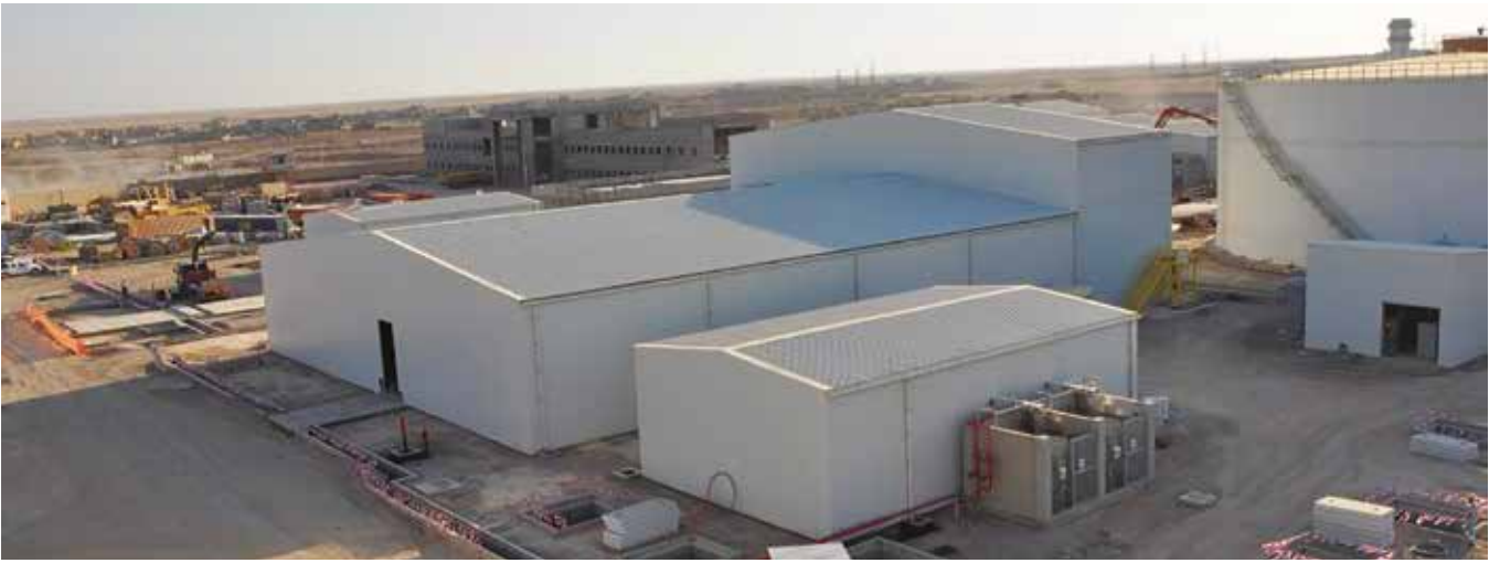
Al Kharirat Power Plant - Irak
