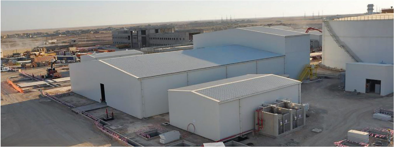
Al Kharirat Power Plant - Irak
