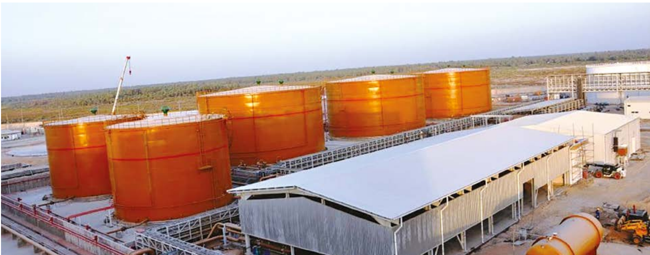
Nainawa Power Plant - Irak
